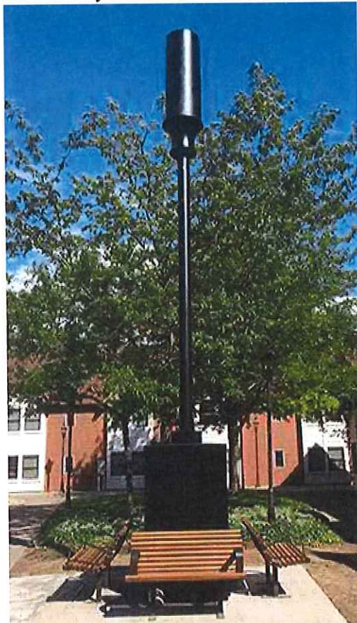
New Pole with Base Equipment Shroud
